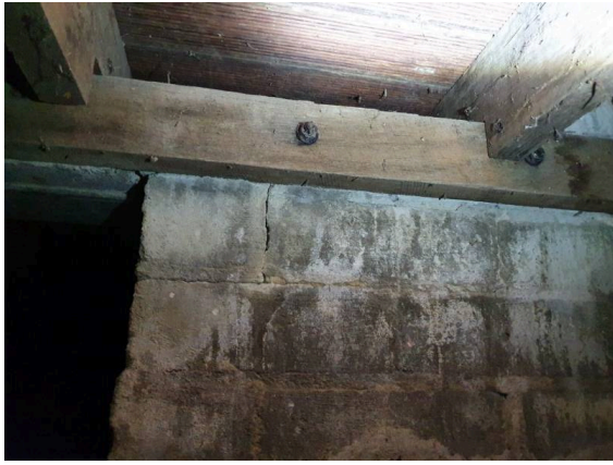
No metal shields on wall in subfloor unit 14
