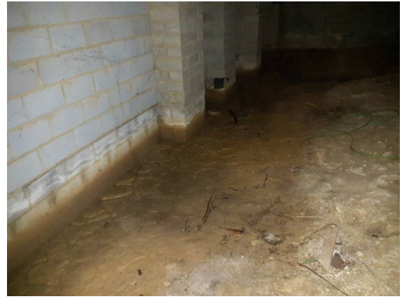
Example of moisture issues in unit 5 subfloor. No water pooling this is evident in most subfloors.
