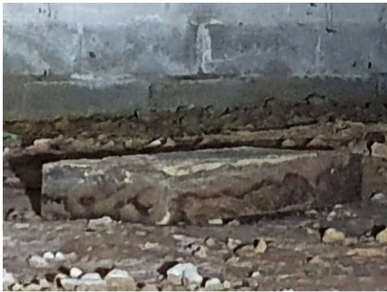
Scrap timber in subfloor unit 8 .
